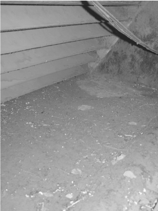
Figure 8. AHU in main building showing thick layer of dust and debris inside.
