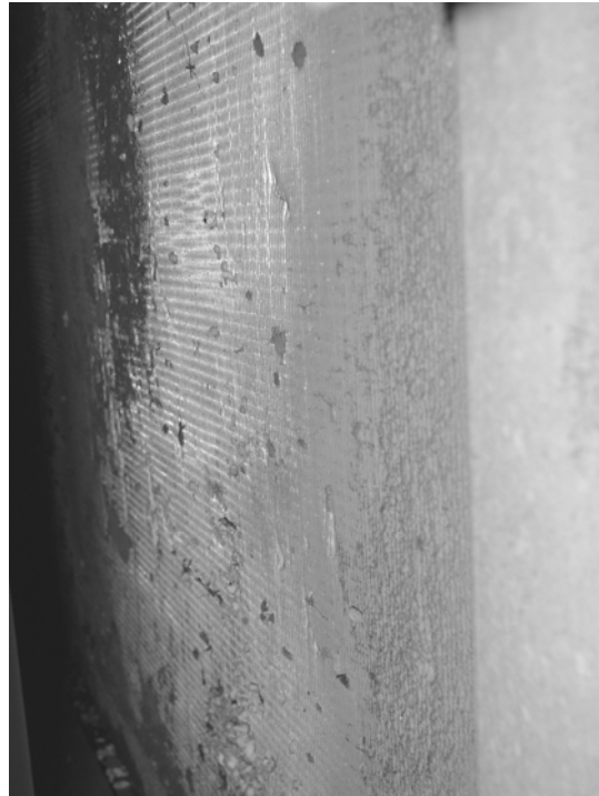
Figure 9. AHU in main building showing dust and debris built up on heating/cooling coils.
