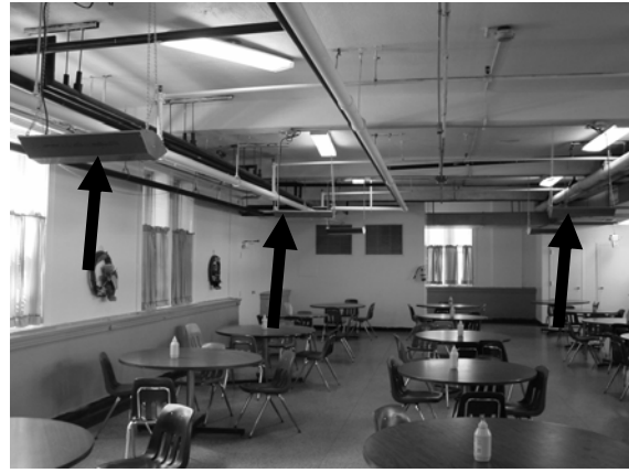
Figure 21. Pendant UVGI fixtures installed in the main building cafeteria.
