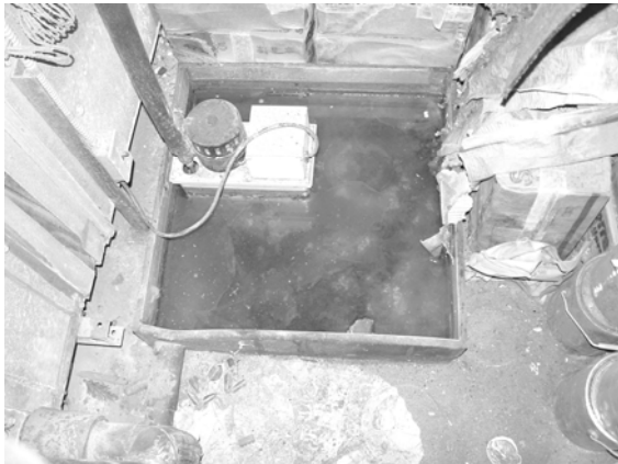
Figure 10. Condensate pan for AHU in main building having inoperable pump. The pan is full of stagnant, dirty water.
