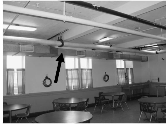
Figure 15. Supply duct work with vents extending along the ceiling of the cafeteria in the main building.
