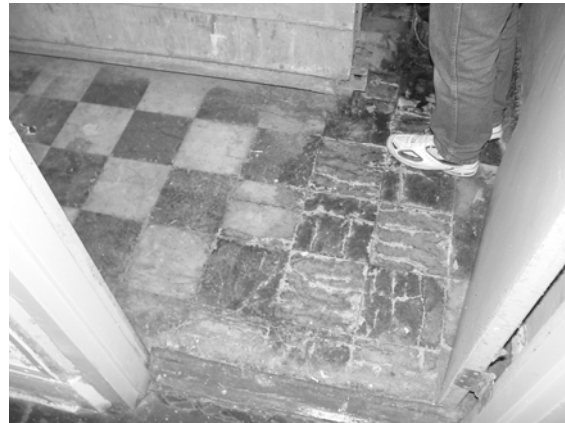
Figure 11. Damage to tile floor where a condensate pan leaked or overflowed.
