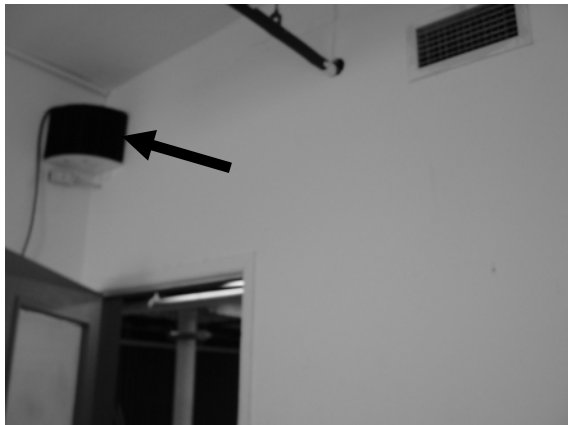
Figure 22. Corner-mount UVGI fixture installed in Nurse Office 1 in the main building.
