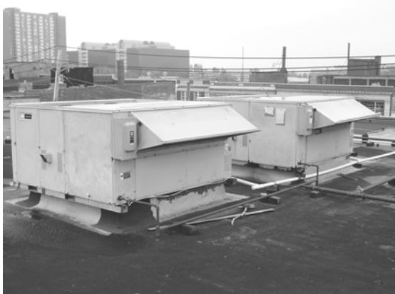
Figure 4. Rooftop AHUs on the annex. Picture shows outside air intakes.
