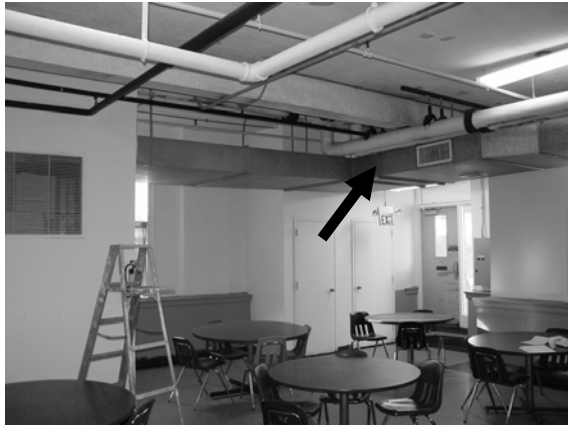
Figure 14. Supply duct work with vents extending from room housing AHU 5 in the main building. A return grille cut into the wall can also be seen on the left.
