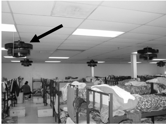
Figure 20. Silent air mover (SAM) UVGI fixtures installed in the annex respite area.
