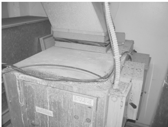
Figure 7. AHU in main building covered with dust and debris.
