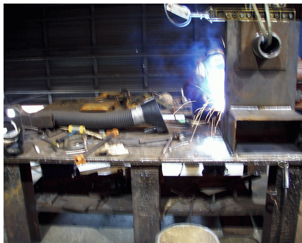
Figure 1: Welding Fume Exhaust
