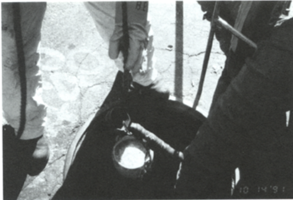
Figure 3. Lowering hot lead ladle into UUV above space where worker is located.
