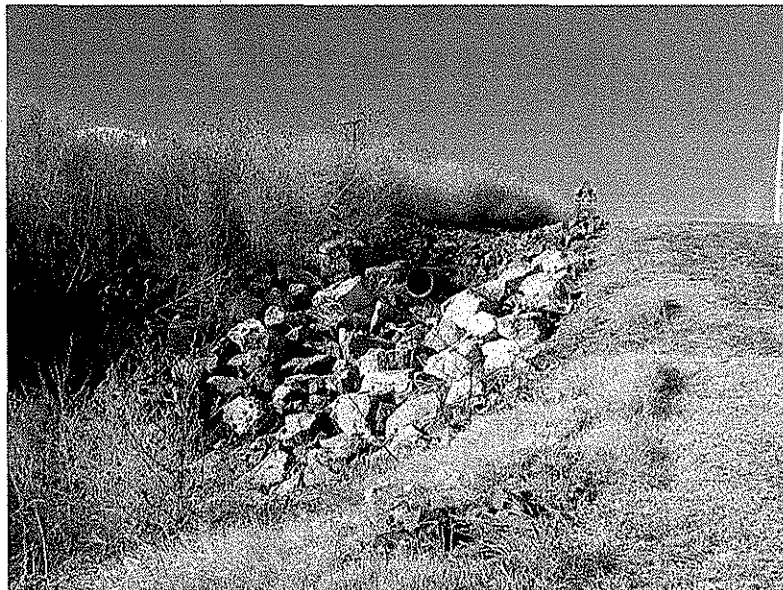
Effluent Discharge Pipe to Tributary to Prairie Dog Creek
