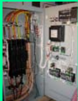
Switchgear, Relays, & Controls
