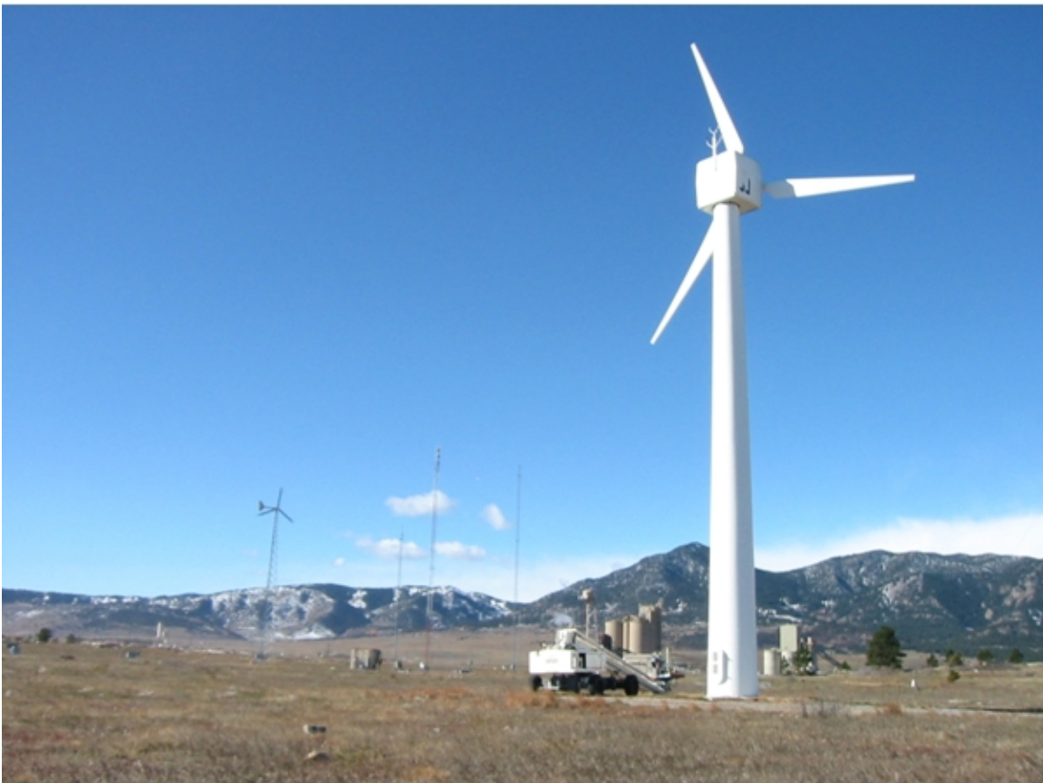
Figure 11. 100-kW wind turbine (NREL 2008)
