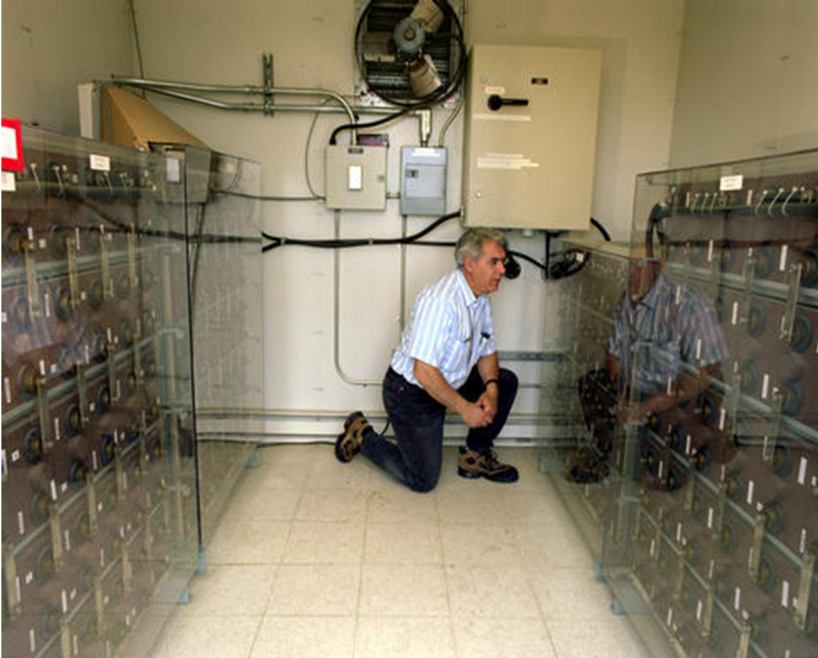
Figure 45. Lead-acid energy storage (NREL 2008)
