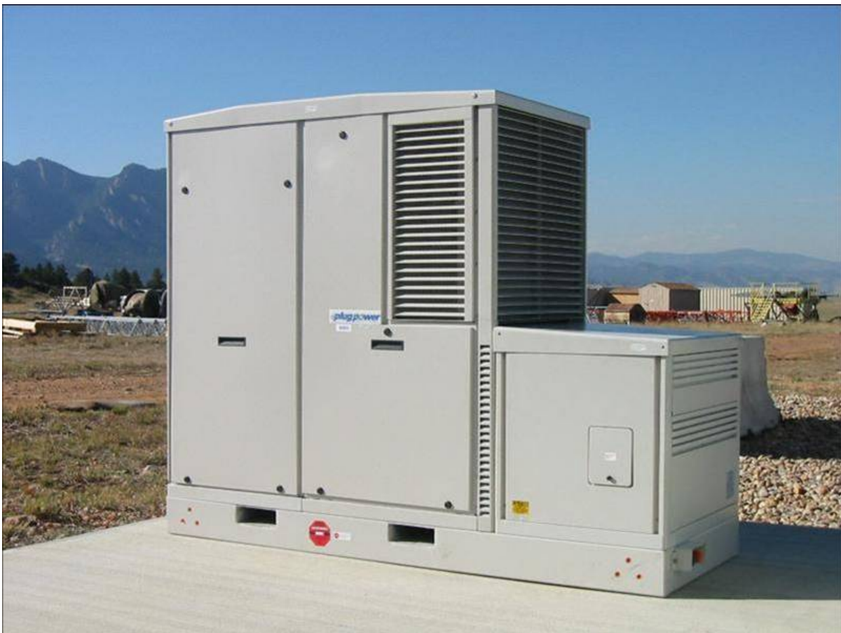
Figure 28. Stationary fuel cell system (NREL 2008)
