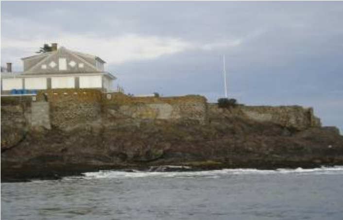
Masonry Wall (Bastion) Storm Damage Repairs, including stairway and landing replacement at the former workshop (left side of the picture).
