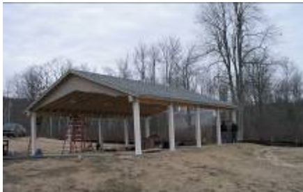
The new Group Picnic Shelter at Lake St. George State Park. A new campground shower building also is being constructed at the park.
