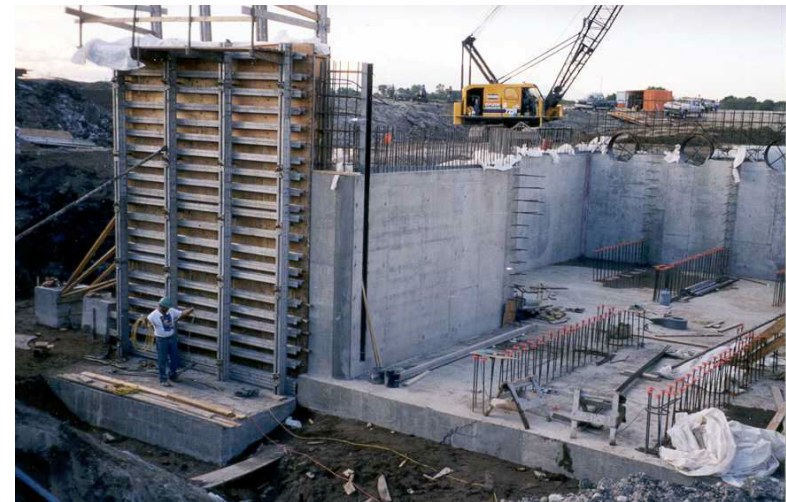
East Ditch Pump Station
