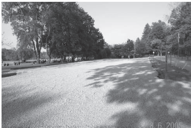
Geoweb was installed to create a parking surface that is pervious at Legion Park, Blair County, PA.
