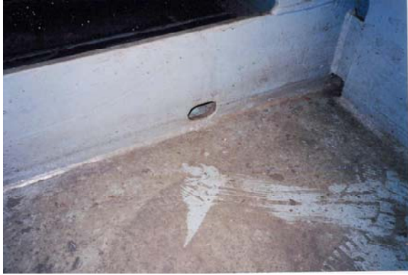
Photo 2.23: An example of poor transverse drainage, a relatively small limber hole with the bottom more than 2cm above the bottom shell.
