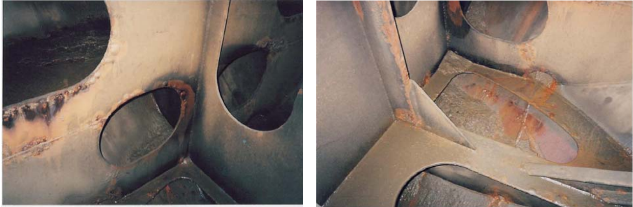
Photo 2.1: Typical connections of internal members and side shell plating in forward part of fore peak tank.
