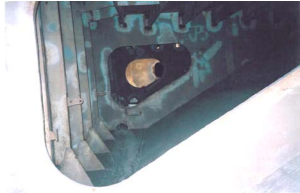
Photo 2.5: An alternative that improves both drainage and cleanliness, longitudinal framing for the sloping plate is in the cargo hold. This permits the tank to also be used for carrying grain.
