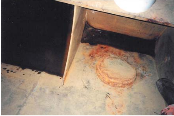
Photo 2.12: Ballast trapped at the forward end of a topside tank by blocked drainage through a bracket at the shell connection.
