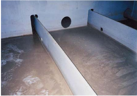
Photo 2.20: Obvious disparity between longitudinal & transverse drainage where longitudinals pass through transverse floor slots.
