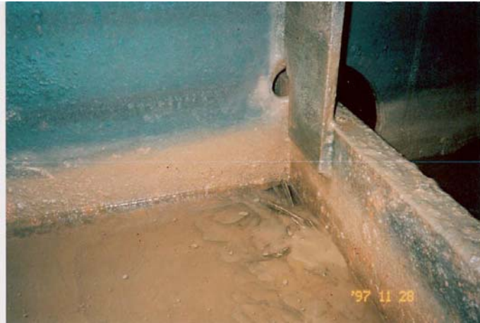
Photo 2.3: Typical connection of transverse floor, longitudinal bottom shell frame and vertical floor stiffener. Note restricted drainage on this side of longitudinal frame, as evidenced by the accumulation of scale and mud.
