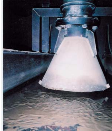
Photo 2.7: Typical bellmouth installation in a double bottom tank.
