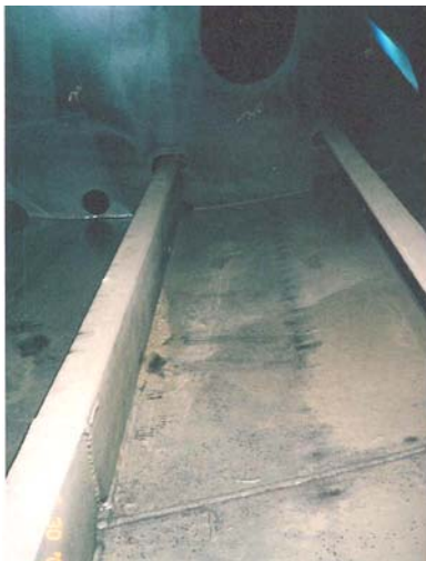
Photo 2.19: Limber holes in longitudinal bilge framing where prefabricated hull units have been joined together. The absence of a continuous frame/shell connection reduces potential accumulation. However the same type of connection to the shell has not been utilized in other locations or members.
