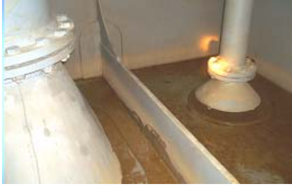
Photo 2.10: Main ballast line and stripping line bellmouths separated by longitudinal shell frame in an existing ocean bulk carrier. Note relatively poor transverse drainage.
