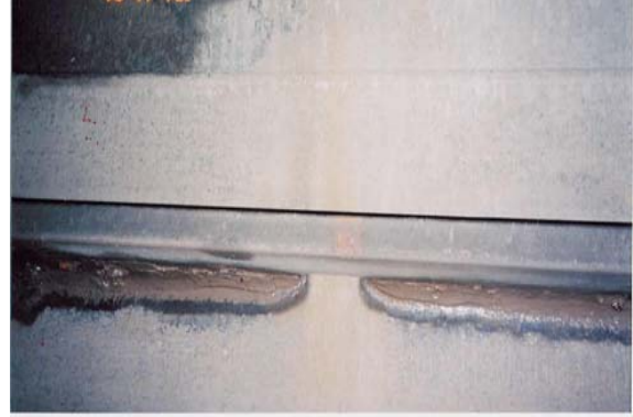
Photo 2.24: By contrast, use of wrap-around welding allows this limber hole through a bottom longitudinal to be open all the way to the shell.
