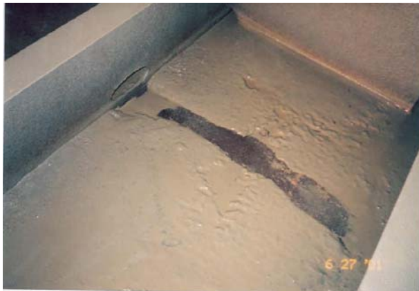
Photo 2.22: Scouring in sediment on the bottom shell is an indicator of flow intensity in the transverse plane in the outboard bays of the double bottom and hopper tanks during the final stages of deballasting, leaving large areas of accumulating sediment between the limber holes in longitudinal shell frames.
