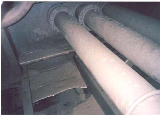
Photo 2.8: Ballast line running through hopper tank showing connection at watertight terminal bulkhead.
