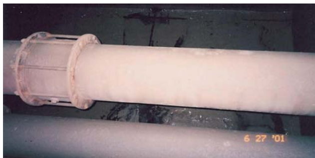
Photo 2.11: Dresser couplings provide watertight connections between pipe sections within the tank. Regular inspections ensure tightness to prevent leakage between tanks and loss of suction to pump from air ingress.
