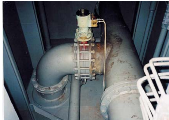
Photo 2.9: Hydraulic lifter and valve to double bottom tank located in lower bulkhead stool. The bellmouth is directly below, 2 meters from the valve.
