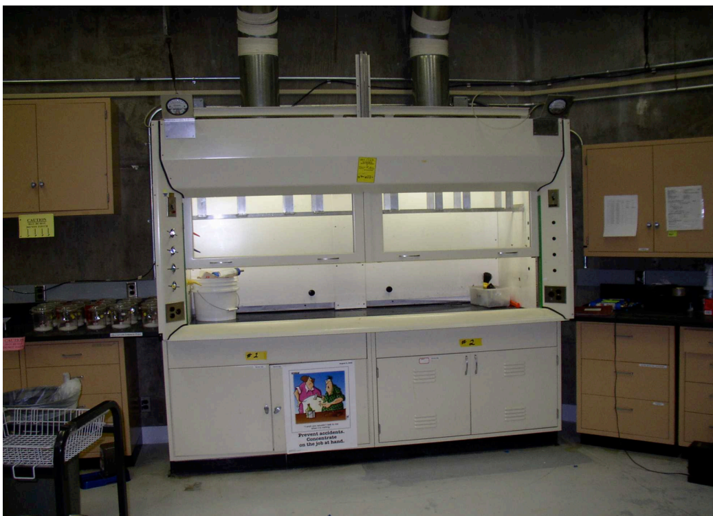
Figure 2-2. Example of chemical use in laboratory hood at LANL.
