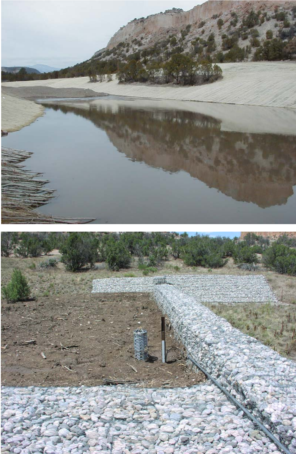
Figure 3.4-3 Photographs of Los Alamos Canyon low-head weir and upstream sediment retention basin on March 30, 2001 (top; view to the west) and July 10, 2006 (bottom; view to the north)
