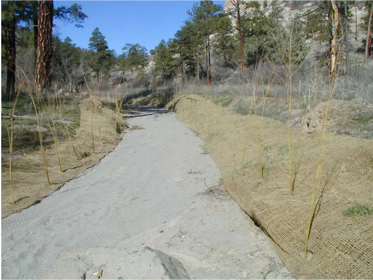
Figure 4.5-1 Photograph of jute mats and willows ( Salix spp. ) used to stabilize banks in Pueblo Canyon, spring 2005 (view to the west)
