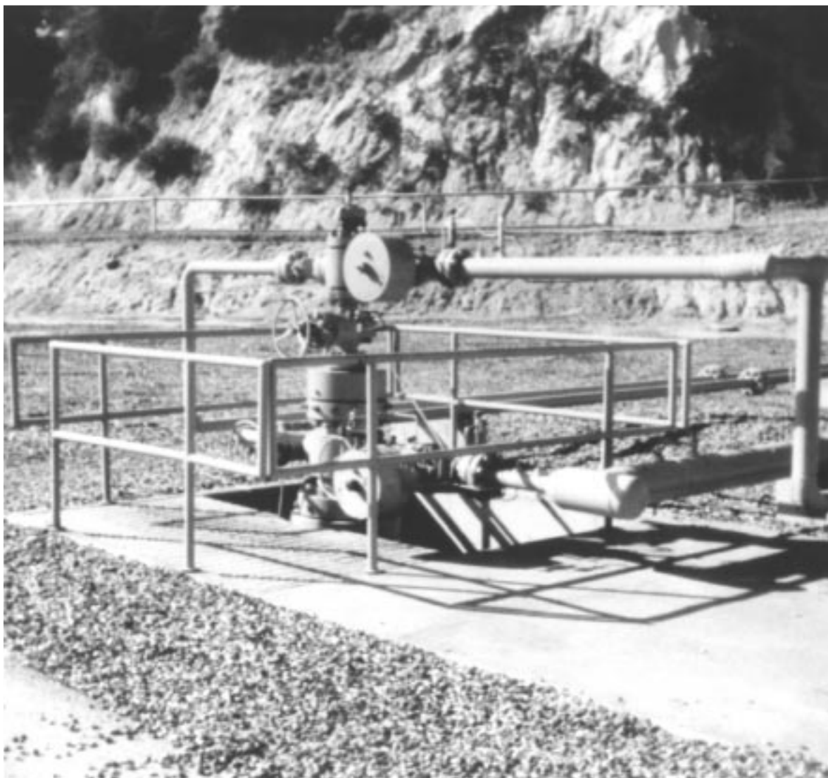
Southern California Gas Company's gas well storage field in Aliso Canyon, California.
