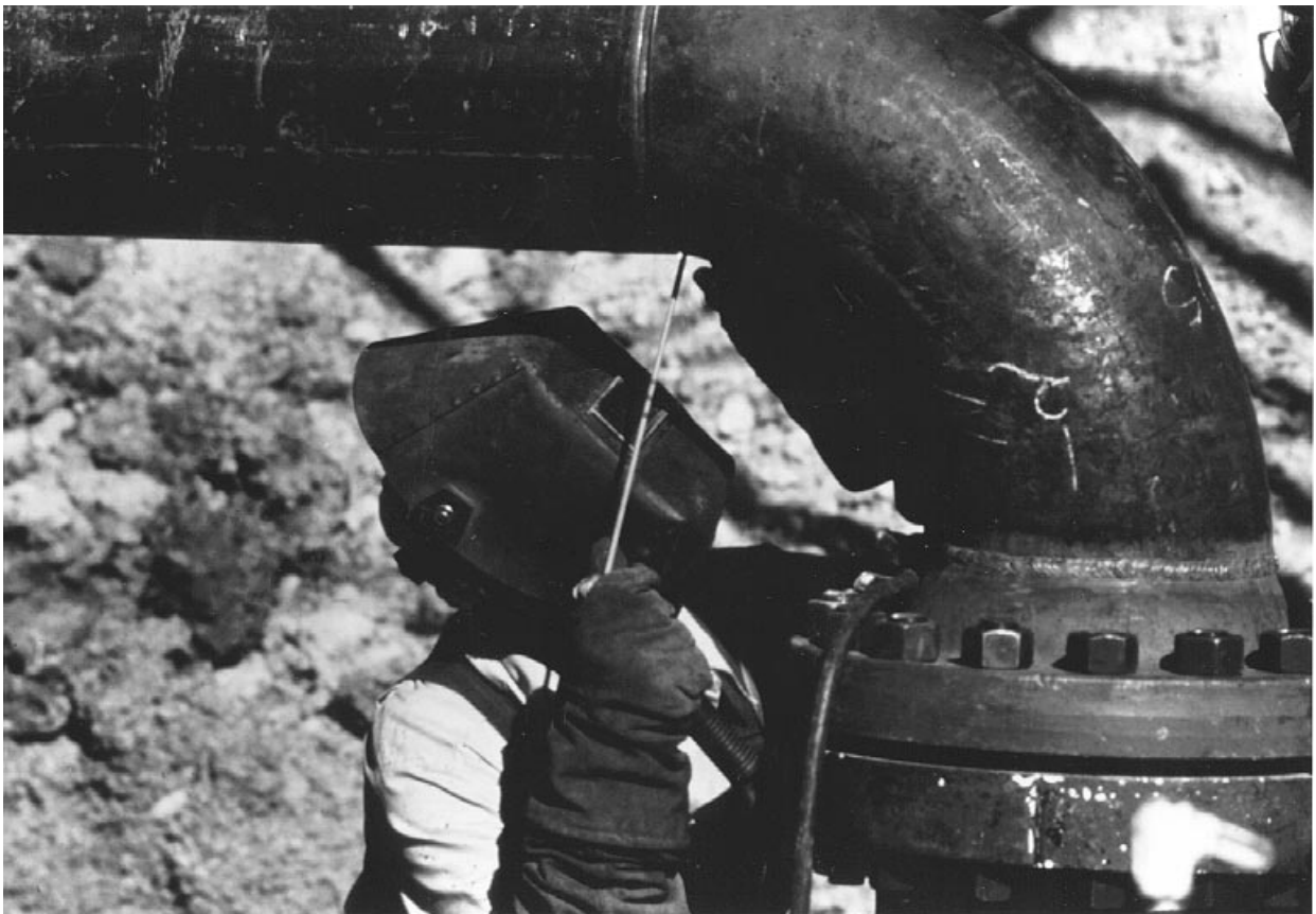
A workman is completing the welding of a 30-inch pipeline section on a natural gas transmission line.
