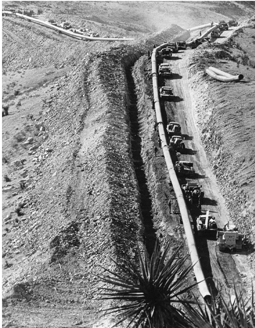
An extensive network of pipeline brings natural gas to consumers.
