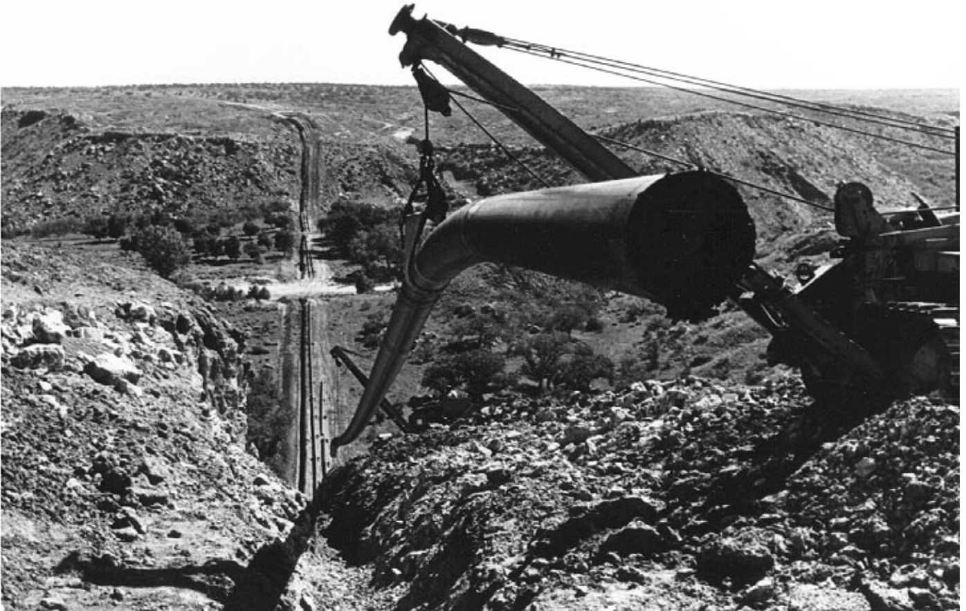
A panoramic view of a natural gas pipeline construction project for Colorado Interstate Gas Company in the Texas Panhandle.
