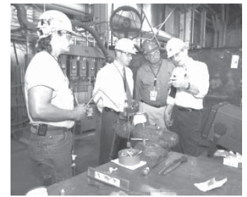
A Savannah River Site Welder Shows Dr. Everett Beckner (Far Right) of the Department of Energy's National Nuclear Security Administration, How He Sets Up his Work For Fabricating and Installing the Internals of the First Two Glove Boxes of the Site's New Tritium Extraction Facility.
