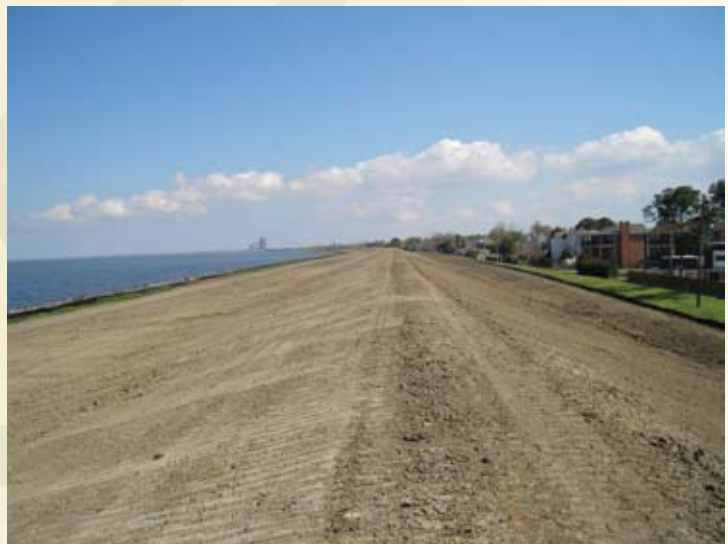
Recent upgrades underway to raise the height of this earthen levee to the 100-year level in the New Orleans area.
