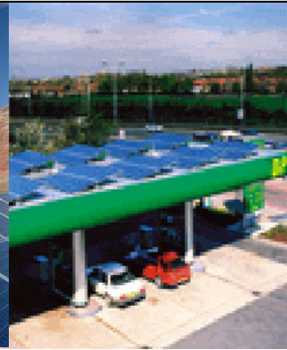
PV panels on rooftop.
