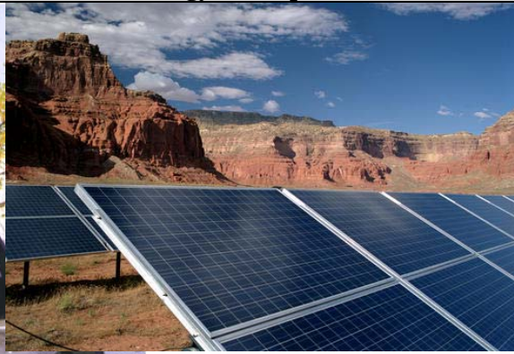
PV solar arrays for larger-scale electricity.
