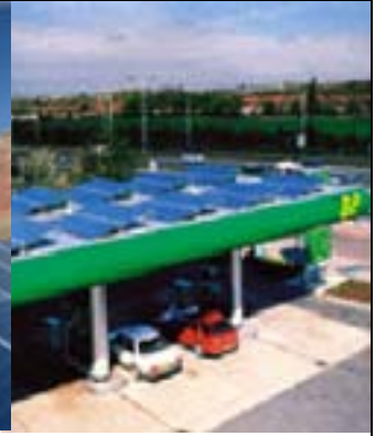
PV panels on rooftop.
