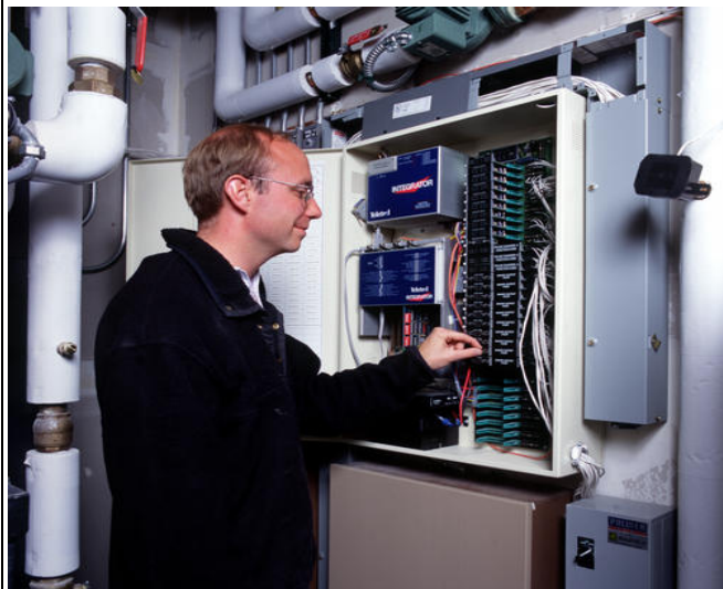
Energy-management system field tests at the Zion National Park Visitor Center (top) and the Bighorn Home Improvement Center complex in Silverthorne, Colorado (bottom), DOE High Performance Buildings Program.
