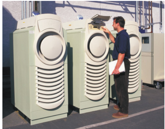
Three 30-kW microturbines are in use at a landfill in Burbank, California, to generate electricity.
