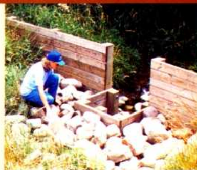
Wood is one of the material choices for relatively inexpensive drop structures that help solve small gully erosion problems.
