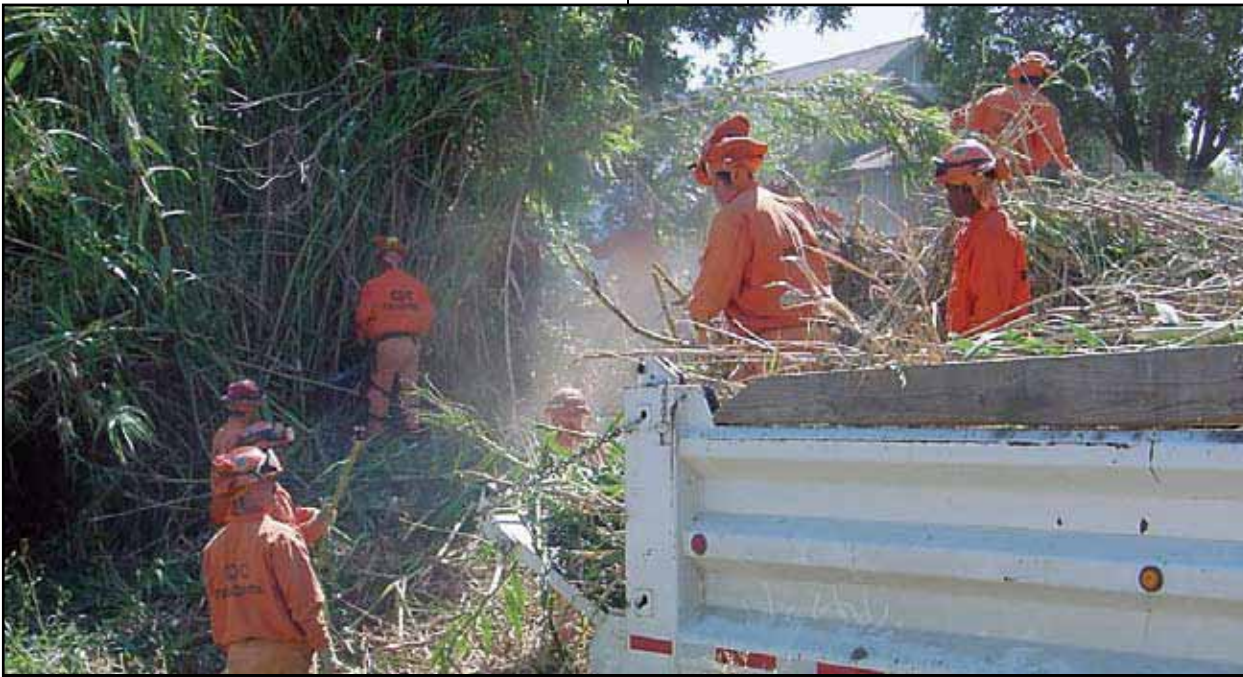
Arundo was successfully eradicated from the Tequesquita Slough watershed in San Benito County. Here, fire crews from the California Department of Forestry remove arundo, which is being cut by chainsaws. The cut arundo is being loaded by hand into a County Public Works dump truck, where it will be moved to a nearby field and burned. Photographer: Ron Ross, San Benito County Weed Management Area
