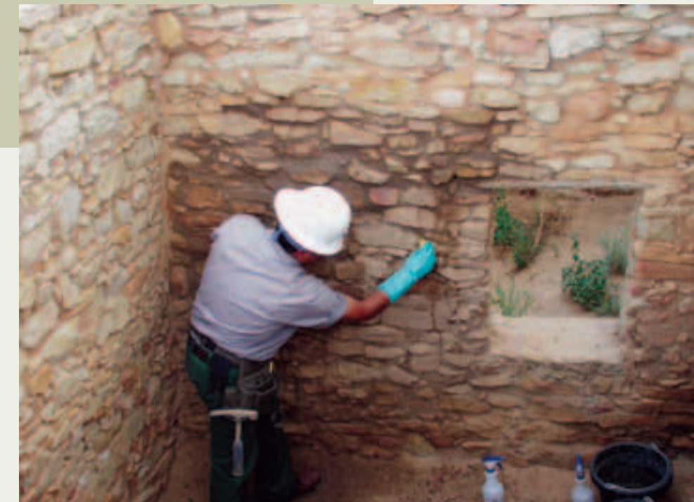
Vanishing Treasures masonry worker treating a gap in a 700-year-old wall at Atsinna Pueblo, El Morro National Monument, New Mexico. (National Park Service)
