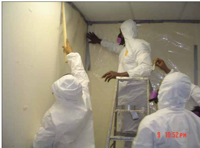
OAI Chicago asbestos training.
