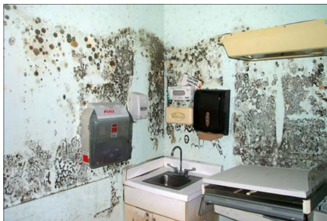
Mold in a hospital after Katrina.
