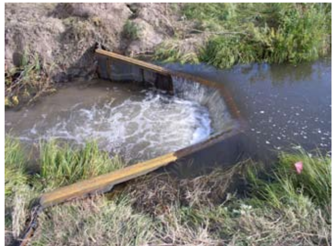
Figure 13–31 Sheet pile vortex weir
