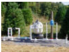
After the water leaves the storage tank it flows to this sand filter system to ensure that no debris pass on to the drip irrigation tubes. Our Marion County Farmer also included an injector at this point to aid in adding nutrients to the water.
