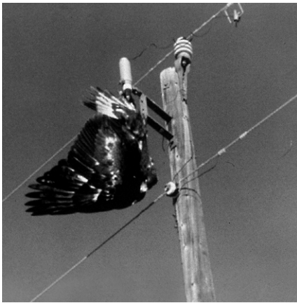
Electric power poles, lines, and equipment represent an electrocution threat to raptors and other migratory birds; agents have forged proactive partnerships with industry to address this problem. USFWS
