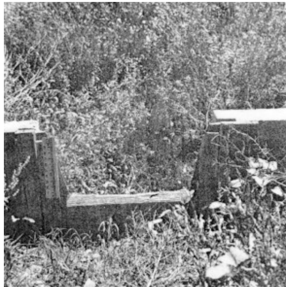
Figure 5-8 -- Poorly maintained weir edge.
