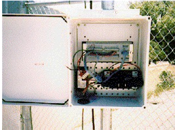
Figure 6-8 -- Programmable battery operated recording unit.
