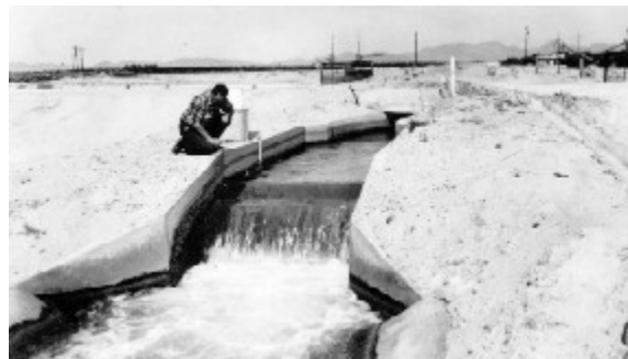
Figure 7-3 -- Suppressed rectangular weir at a canal drop.
