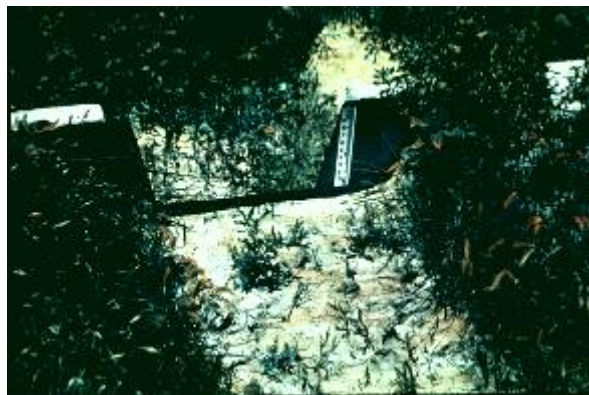
Figure 5-7 -- Sediment deposits in weir pool.
