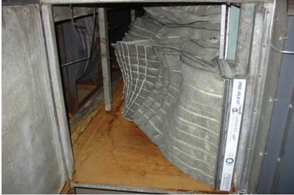
Figure 7. Rust caused by standing water in SF 101 at the DRMC 400 East facility. The excess condensate during periods of rain/high humidity typically saturates the filters. This is typical of many AHUs at 400 East.
