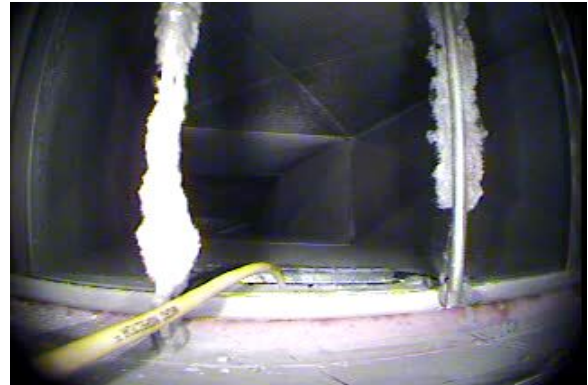
Figure 10. Snapshot from video examination of the inside of the return duct above the ceiling in the neonatal intensive care unit (NICU) on the third floor of the DRMC 400 East facility. The ductwork showed visible accumulations of lint.
