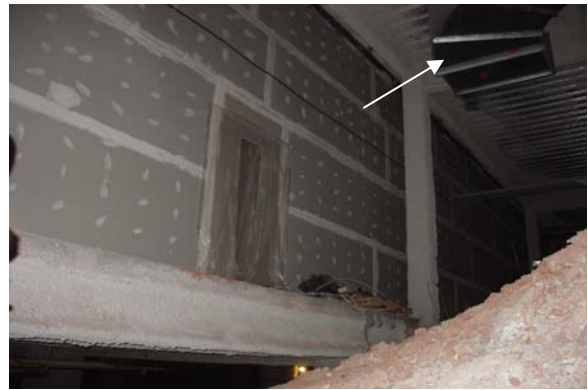
Figure 4. Ventilation supply ductwork from AHU2 running through a portion of the crawlspace under the DRMC River Road facility.
