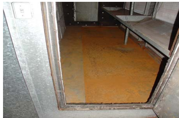
Figure 6. Rust caused by standing water in SF 101 at the DRMC 400 East facility. The standing water results from an excess of condensate collected during periods of rain/high humidity that overwhelms collection basins.
