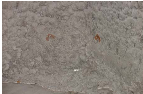
Figure 12. Pile of lint inside return fan (RF) 202 at the DRMC 400 East facility. Lint is easily removed by ventilation filters and not recirculated back into the hospital.
