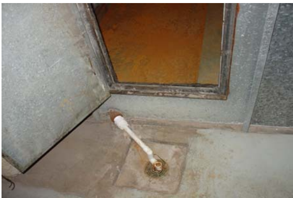
Figure 5. Drain for SF201 at the DRMC 400 East facility does not provide sufficient drop for proper drainage of excess condensate collected on the cooling coils. This is typical of many AHUs at 400 East.
