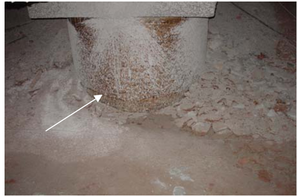
Figure 2. Column support with cardboard form in place in the crawlspace below the DRMC River Road facility. There were signs of past water incursion (arrow) but no visible mold.
