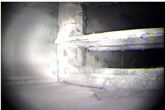
Figure 11. Snapshot showing accumulation of lint inside of the return duct above the ceiling in the neonatal intensive care unit (NICU) on the third floor of the DRMC 400 East facility.
