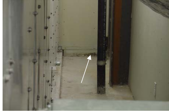
Figure 8. Water damage and small amount of mold (arrow) in rooftop air handler room for AHU 4 th West. The AHU has a ducted air return, so the room does not serve as a return air plenum.
