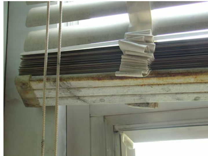
Figure 16. Rust, dirt, and possible mold on an aluminum blind in the High School library.
