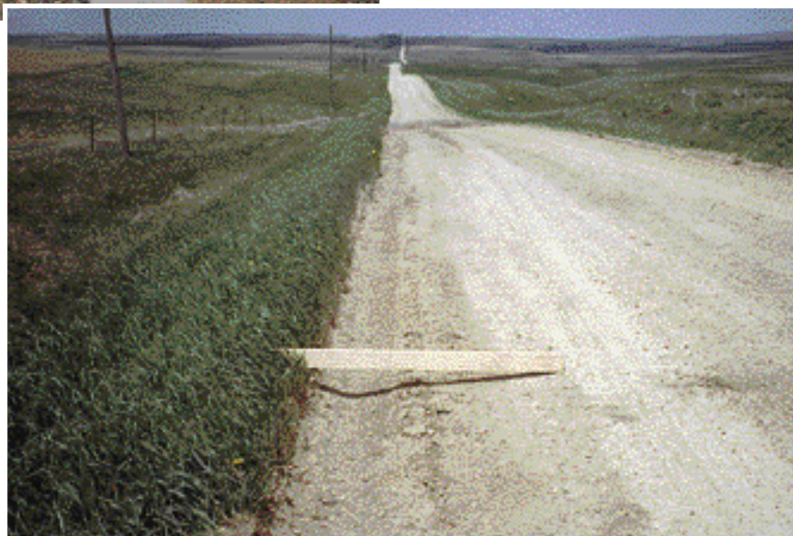
Secondary ditch over six inches deep.
