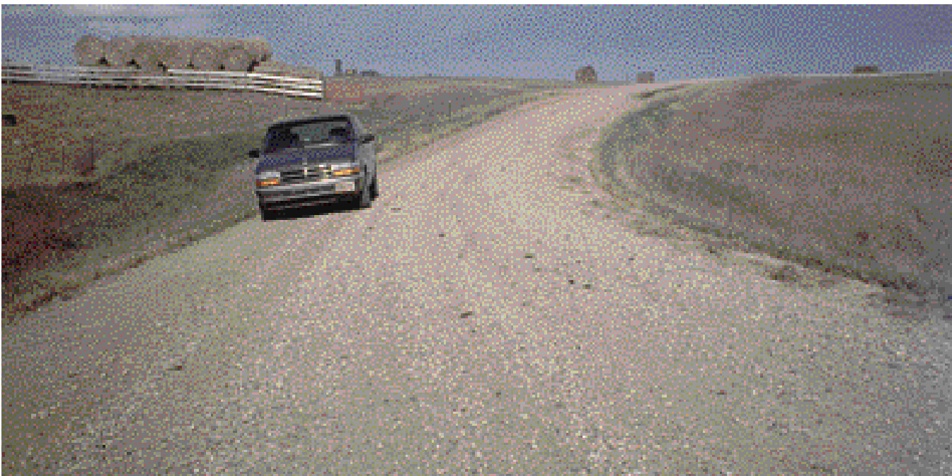
This photo shows lack of superelevation which can lead to accidents.
