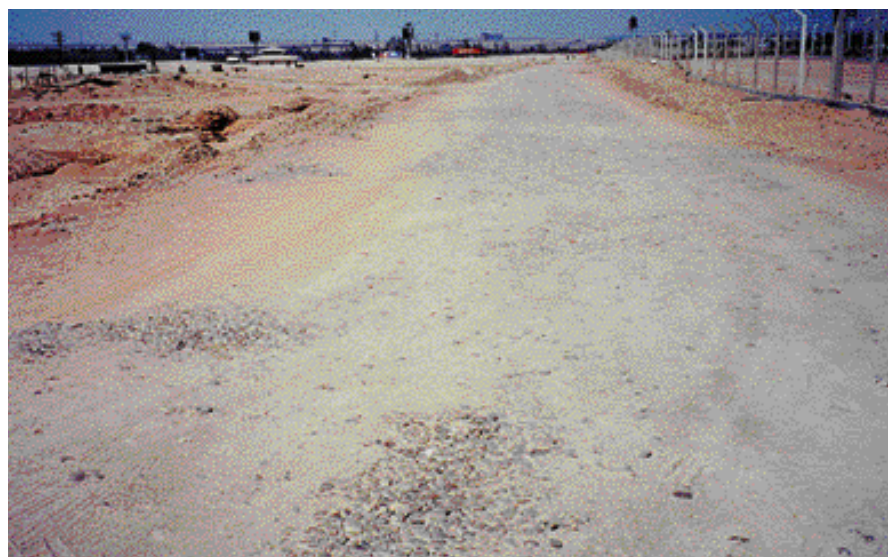
This road is located about 50 miles from Cairo, Egypt. It displays segregation problems in several spots. (Photo courtesy of Ali Selim, SD LTAP, USA)
