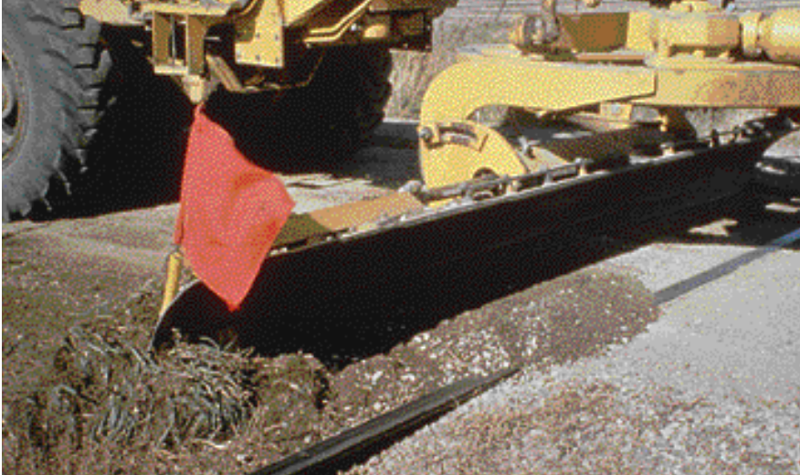
Grader working at a rural railroad crossing. The material that has been pushed into the flangeway should be removed.
