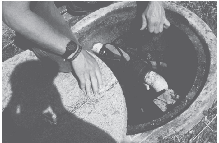
All systems at Stinson Beach have tank risers, lateral valves and risers, and inspection ports. The pumps also have an elapsed time meter and a dose counter to verify the wastewater loading to the bioreactor in this recreational community.
