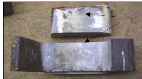
Figure 2. Autopsy of IJ Shows Benefit of using Flexible Material at End Post. Arrows Show No Rust at End Post Fastener Types
