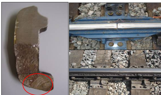
Figure 4. Joint Bar with Fatigue Crack. Removed after 75
