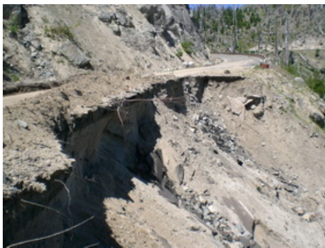
Road damage at mile post 8 on Forest Road 99, July 2008
