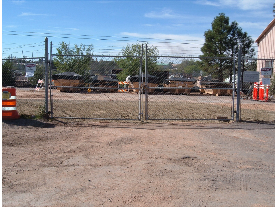
Figure B-15 Excavated area was restored with base course after backfilling was completed. Note five roll-off waste bins with covers that contain petroleum-contaminated soil removed from northwestern corner of SWMU 61-002.
