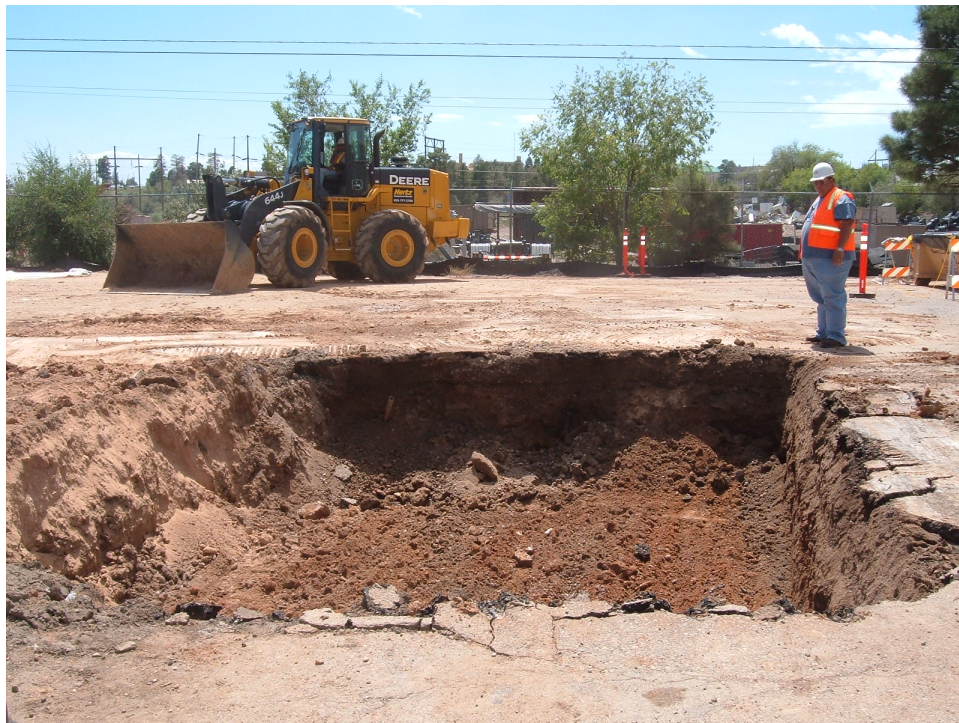
Figure B-8 Excavated area at SWMU 61-002 near access gate (view looking south toward the Los Alamos County Landfill)
