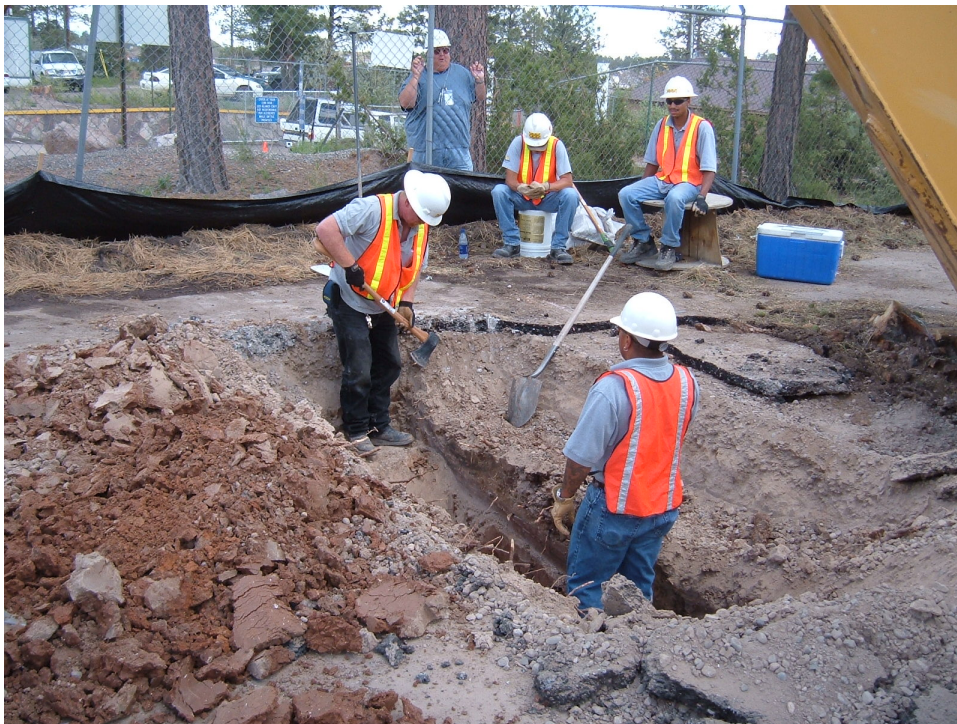
Figure B-6 Potholing before excavation at SWMU 61-002. Pothole dug to find water line shown on excavation permit map near northeast corner of property. No water line was found after hand digging to 6 ft bgs.
