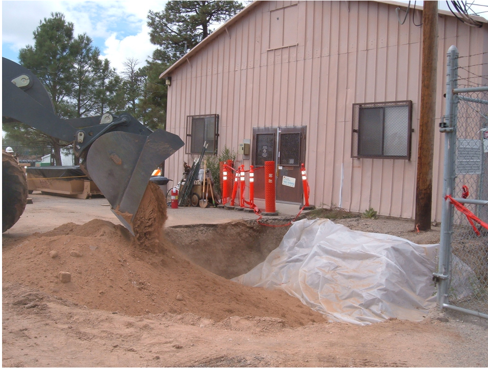
Figure B-13 Backfilling area where petroleum hydrocarbon contamination was found in northwestern corner of SWMU 61-002 (Building 61-23 in background)
