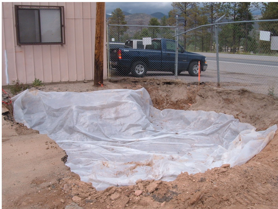
Figure B-12 Installation of plastic layer before backfilling with clean fill in northwestern corner of SWMU 61-002 where petroleum hydrocarbon contaminated soil was found (Building 61-23 in background)
