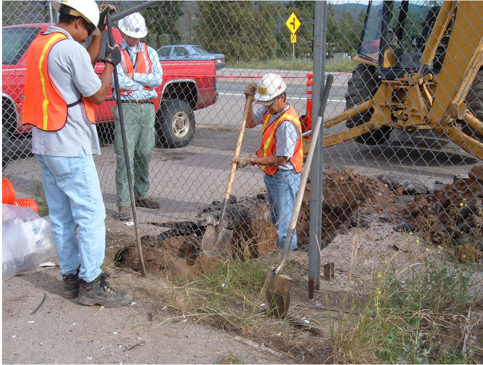
Figure B-5 Potholing before excavation at SWMU 61-002. Pothole dug for locating buried electrical cable near the northern fence line.
