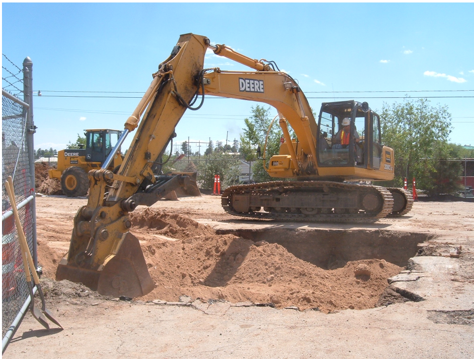
Figure B-10 Backfilling excavation with clean fill using trackhoe at SWMU 61-002 near access gate area
