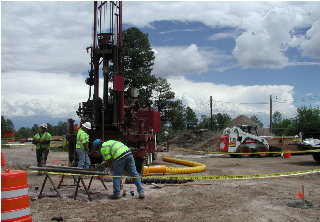
Figure B-17 Installation of borehole location 61-26621. Note exhaust fan to disperse VOC vapors away from borehole.
