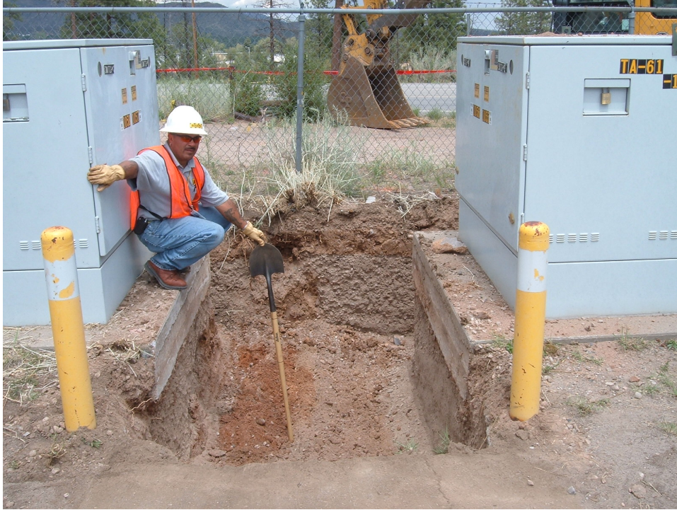
Figure B-9 Hand excavating around electrical utility boxes at SWMU 61-002 (view looking north toward East Jemez Road)
