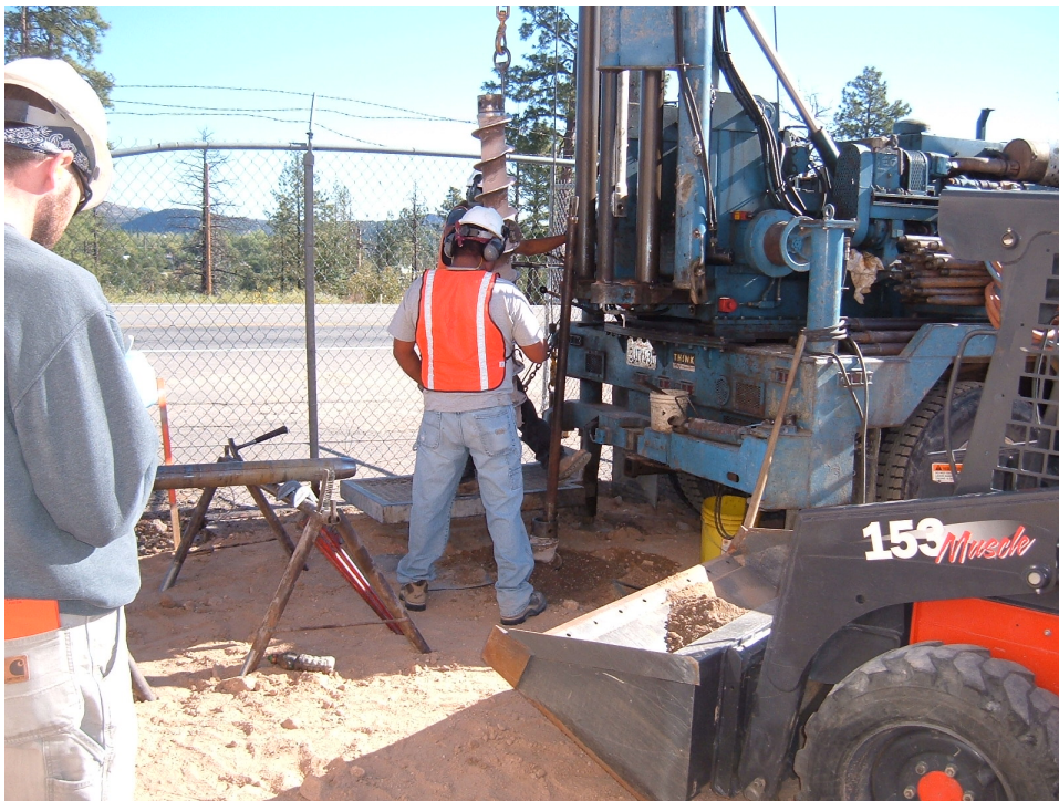
Figure B-14 Drilling at SWMU 61-002 (location 61-24352) near northern fence line to characterize petroleum hydrocarbon contamination
