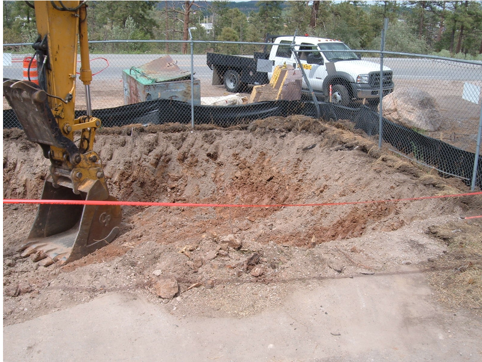
Figure B-7 Excavation activities at SWMU 61-002 started from northeastern corner of site, as shown in this photograph, and continued eastward in a 20-ft swath along the northern fence line.
