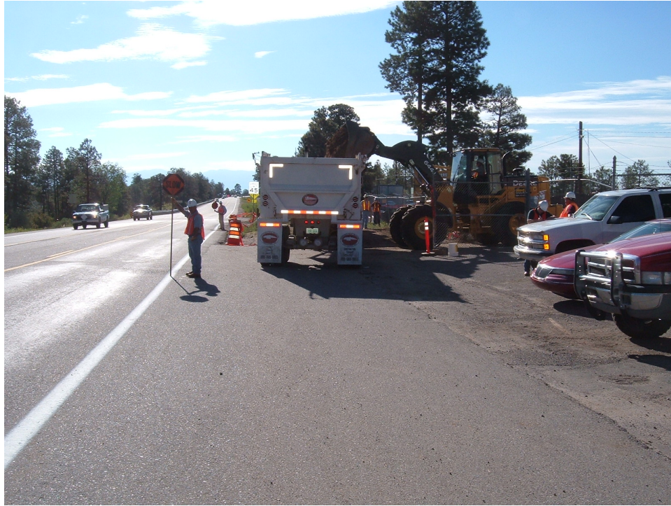
Figure B-11 Truck loading at SWMU 61-002 along West Jemez Road. Material was hauled to Waste Control Specialists in Andrews, Texas for disposal.
