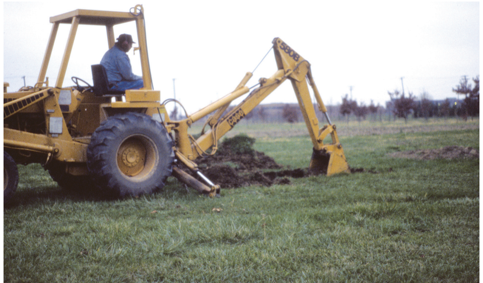
Figure 12. Confirmation of the soil to be used for wastewater treatment is made in a soil pit. An excavation, large enough for a person to safely stand in is made to enable the evaluator and the regulator to make detailed observations, in situ, of the soil in consideration. Since soil pits disturb the site for wastewater treatment, pits are excavated just outside the planned treatment area.
