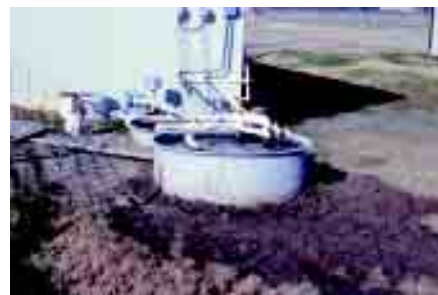
Pit recharge systems are used to improve air quality by reducing gaseous odors.
