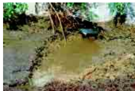
Drain line from sediment basin
