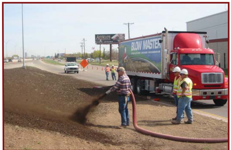
Figure 2: Grass seed and compost being applied as a compost blanket for erosion control and revegetation of a road right-of-way.
