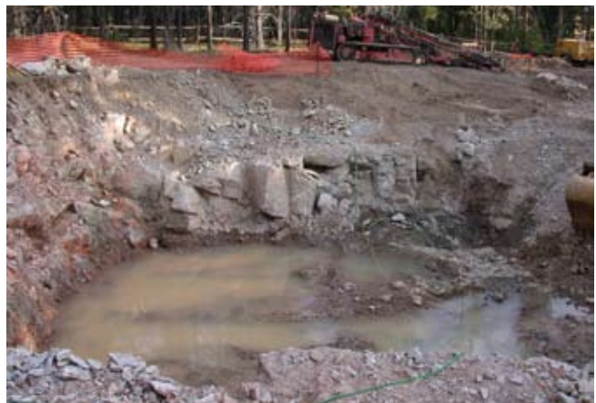
Figure 8. Natural fractures exposed during an excavation for the Norris water treatment plant, September 2003. The water level in the excavation is about ( \pm 1 foot) equal to the water level of the nearby Gibbon River.
