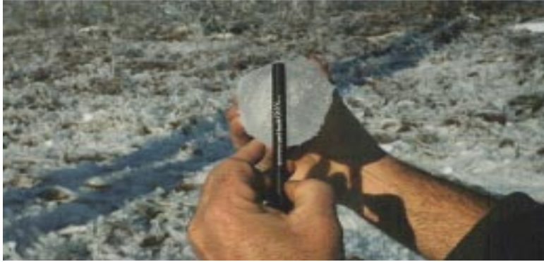
l. ~0.9 in. accreted on a conductor at about 200 ft east of Deblois, Maine (photo Larry Billings, Bangor Hydro).
