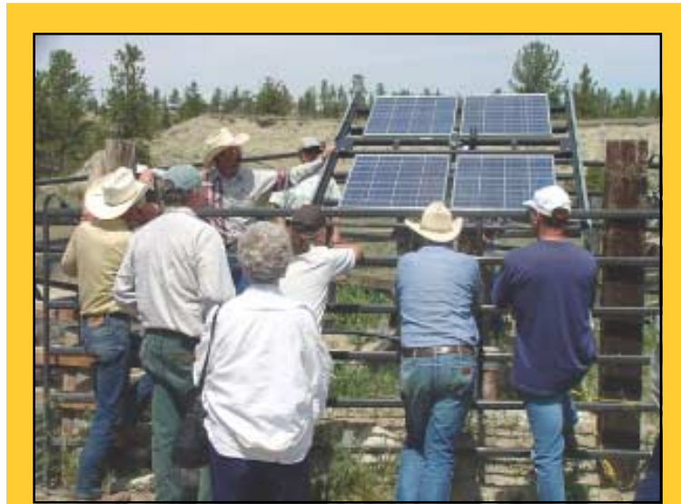
A tracking PV array replaced an old and unreliable windmill on the Ballard Ranch near Lavina, MT.
