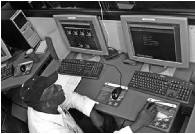
Power plant operators spent most of their time monitoring systems for problems.
