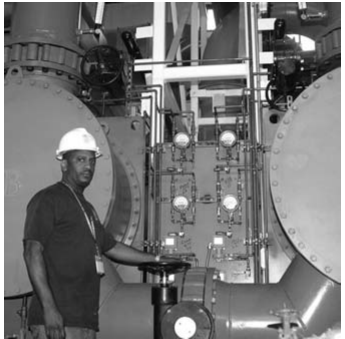
Stationary engineers monitor boilers and make necessary adjustments and repairs.
