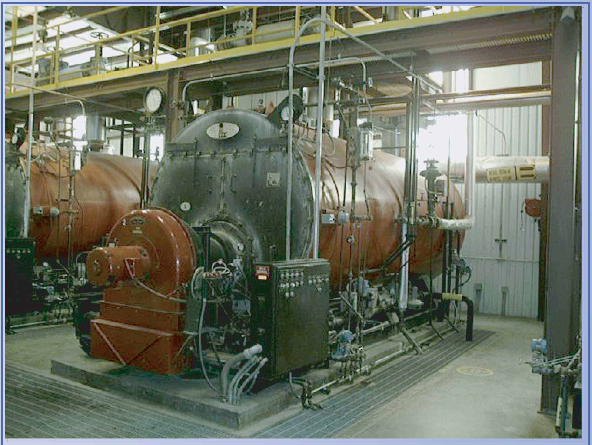
Boiler at Technical Area 21
