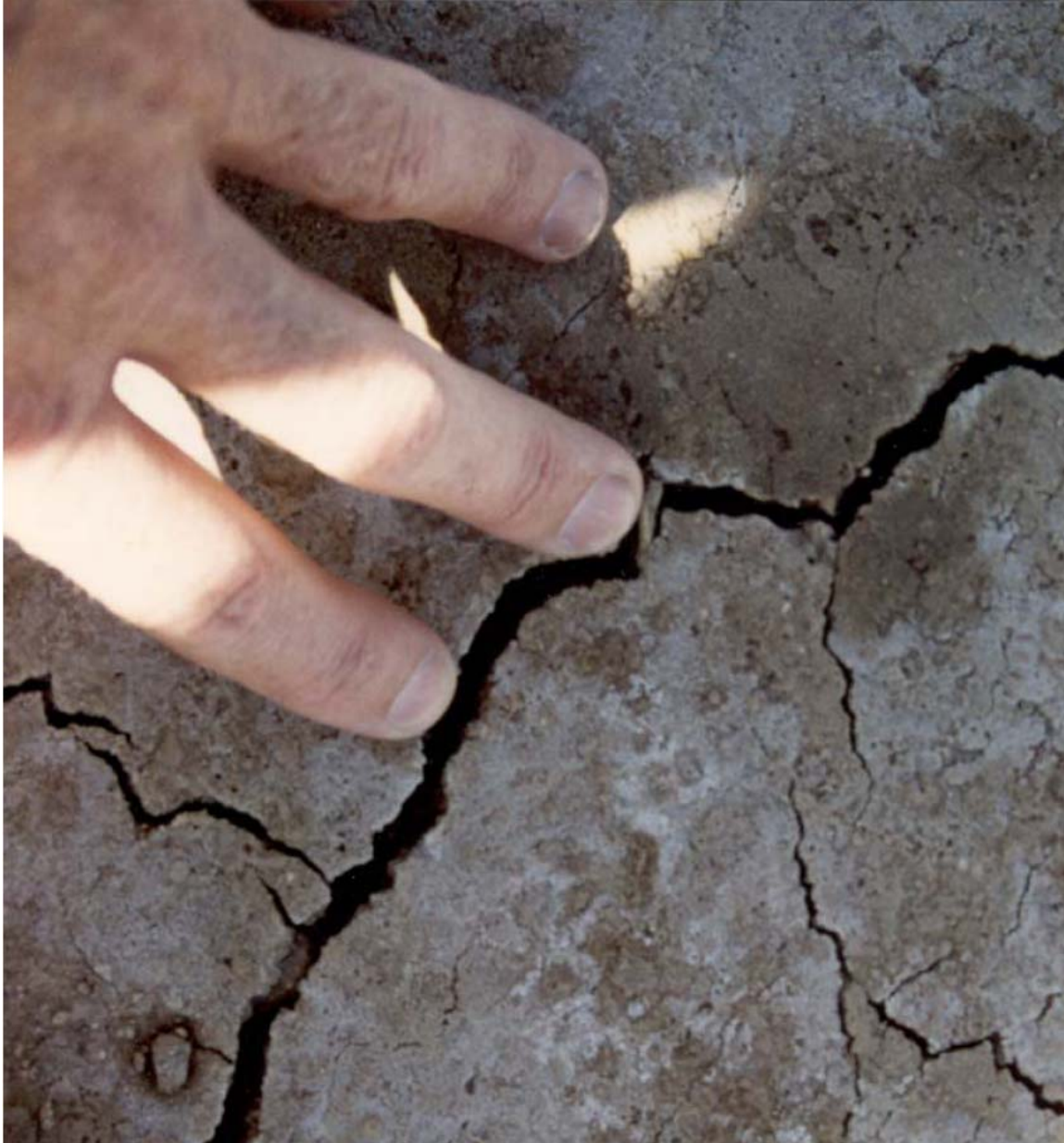
Figure A-2.0-2. Desiccation cracking in clay barrier layer
