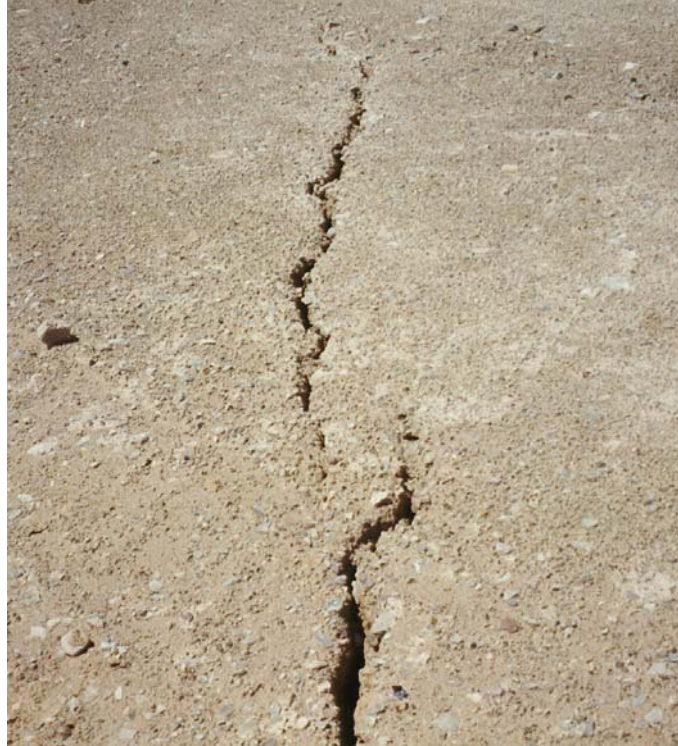
Figure A-2.0-3. Longitudinal cracking due to differential settlement
