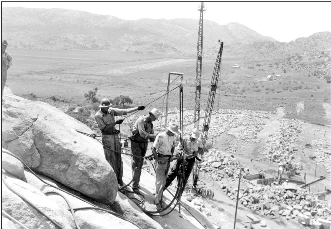
Drilling crew at work on rock face of mountain above quarry bench, July 9, 1941. Below, granite blocks are separated by size and shape for use as facing or riprap in the construction of Altus Dam (National Archives and Records Administration 1941a).
