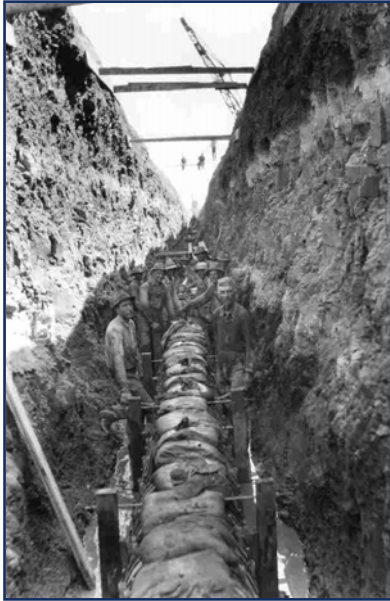
Construction of the redwood pipeline that carried water from the original Lake Altus Dam south to the city of Altus, circa 1927. Photo courtesy of the Museum of the Western Prairie, Altus, Oklahoma. Used with permission.
