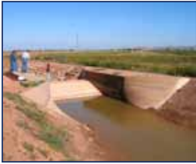
View of a recently installed measurement structure in the West Canal, October 13, 2004. This broad-crested weir allows more accurate measurement of flow from the Main Canal into the West Canal. Photograph courtesy of Bureau of Reclamation, Austin, Texas.
