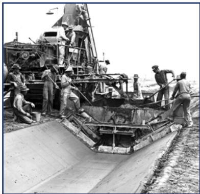
View of freshly laid plastic soil-cement canal lining in West 11.5 Lateral, May 5, 1947. The paver and mixer traveled at a rate of five feet per minute while soil-cement material was distributed into the hopper by hand (National Archives and Records Administration 1947a). This and other low-cost liner applications were used to minimize water loss in high seepage areas of the canal and lateral system.
