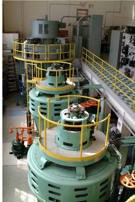
Shoshone is the region's oldest powerplant placed in service in 1922. Original units in the foreground are no longer used and have been replaced by a new one in back.
