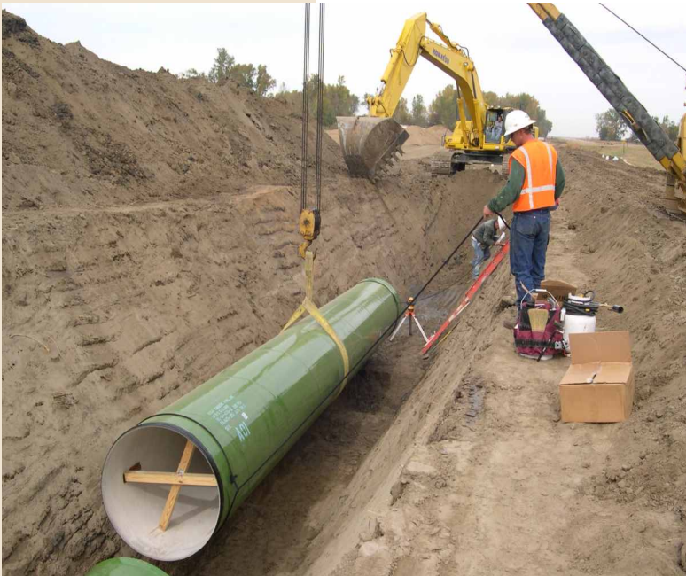
Pipe being laid in the trench on the Lewis and Clark Project in southeastern South Dakota.
