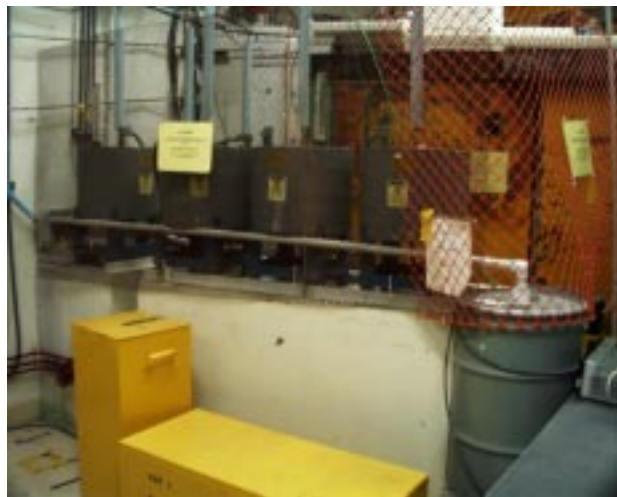
Figure 7-1. Mercury Shutter System at LANSCE. Storage tanks (4) and helium filtration (lower right), with piping system (blue pipes from four storage tanks). Tanks store mercury delivered through the blue pipes as the shutters for the neutron beam are opened by pressurized helium, which is filtered for residual mercury.
