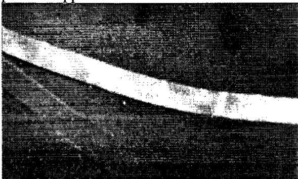
Figure 1 - Infrared thermogram display indicating damaged electric cable insulation
