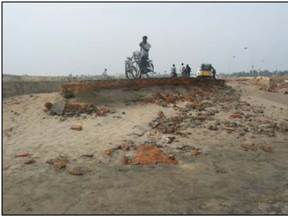
Figure 4: Intense erosion of front portion of beach road, facing to the sea coast at Nagapattinam beach.
